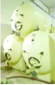
5.000 Litres Steel Pressure Tank
