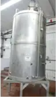
8.000 Liter Storage tank / Agitator tank in V2A
