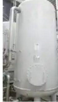
9.000 Liter Storage Tank / Pressure Tank
