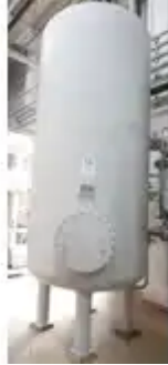
6.800 Liter Storage Tank / Pressure Tank
