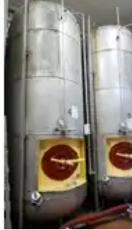
5 750 liter Sparkling Pressure Tank / Sparkling Cooling Tank 8 bar
