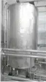
5.000 Liter Storage Tank / Agitator Tank in V2A
