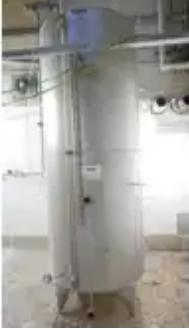
3.400 Liter storage tank
