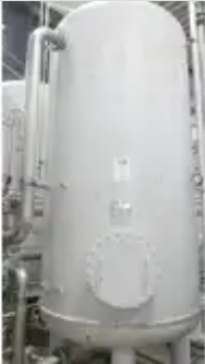
9.000 Liter Storage Tank / Pressure Tank
