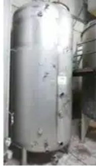
3.000 Litres Storage Tank
