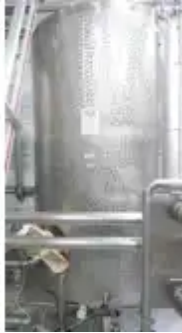
5.000 Liter Storage Tank / Agitator Tank in V2A
