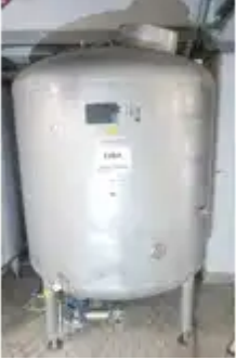
3.000 liter acid tank/ storage tank vertical in V2A
