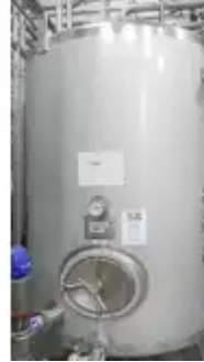
4.721 Liter Lye CIP Tank in V2A
