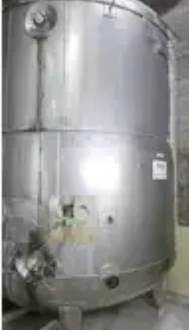
7.100 Liter storage tank with cooling jacket and insulation
